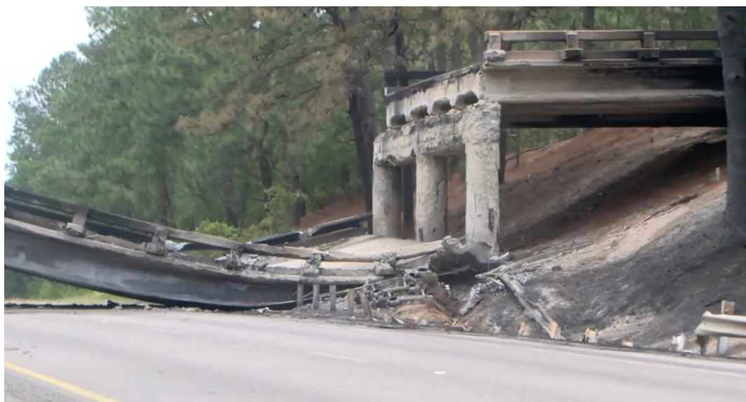
FIGURE 8: OLD VAUCLUSE ROAD BRIDGE COLLAPSE, AIKEN COUNTY, SC
