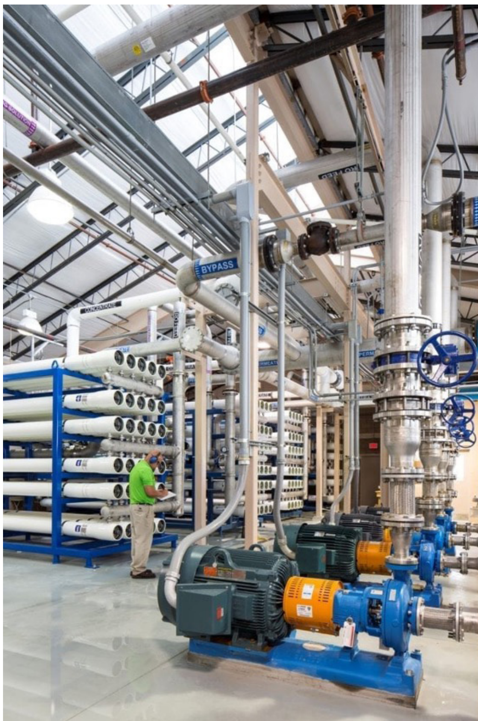
FIGURE 1: HILTON HEAD REVERSE OSMOSIS TREATMENT FACILITY [15]
