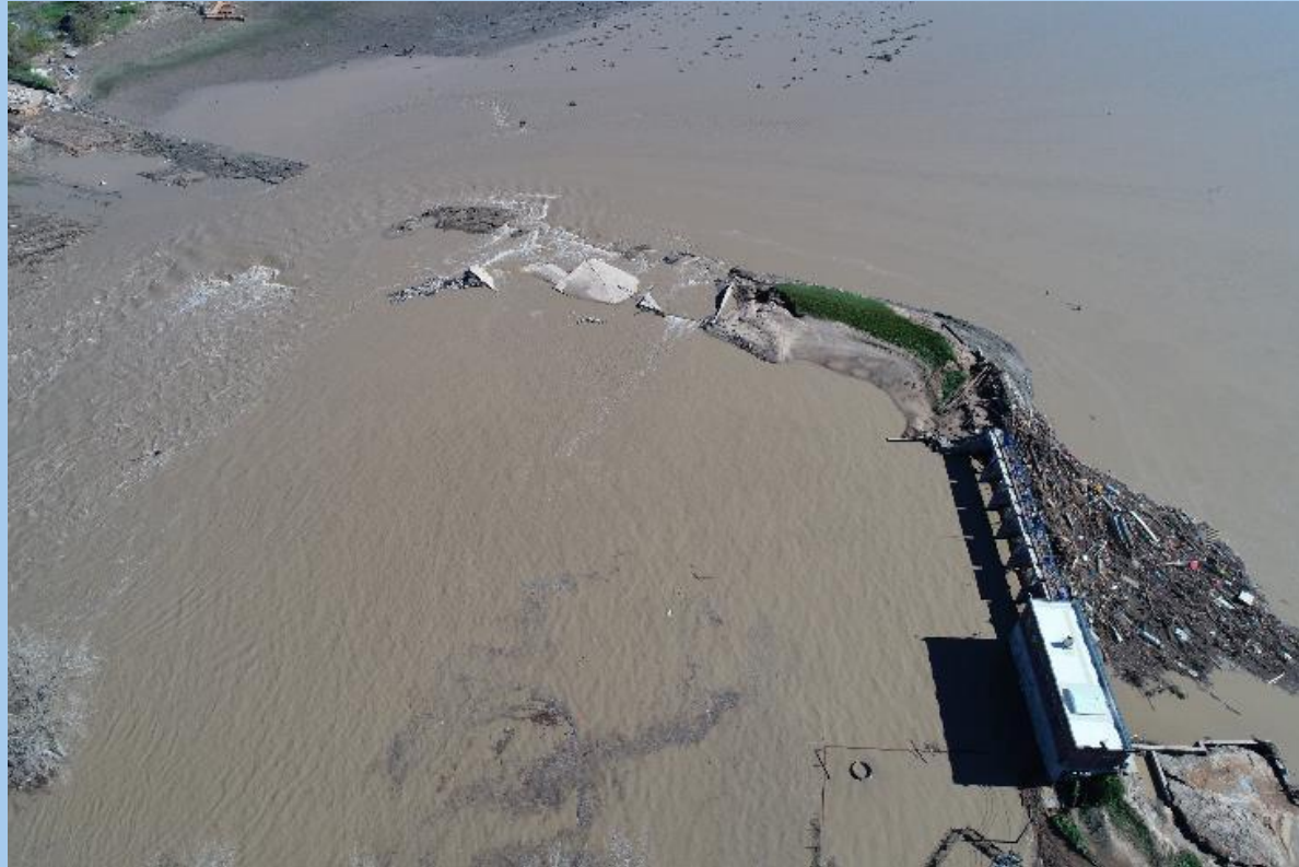
OVERTOPPING OF SANFORD DAM
