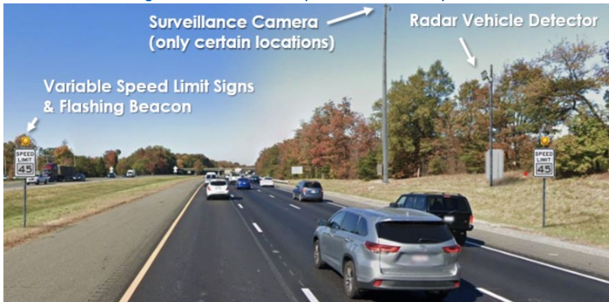
Figure 9: I-95 Variable Speed Limit (VSL) System
