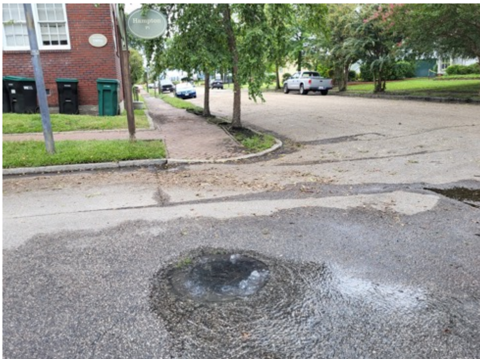
Figure 6: Sanitary sewer overflow following tropical storm Ophelia.
