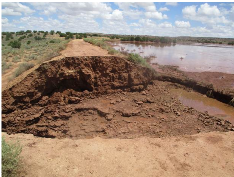
Photo 3: MILLET SWALE DAM POST-FAILURE, JULY 2021
