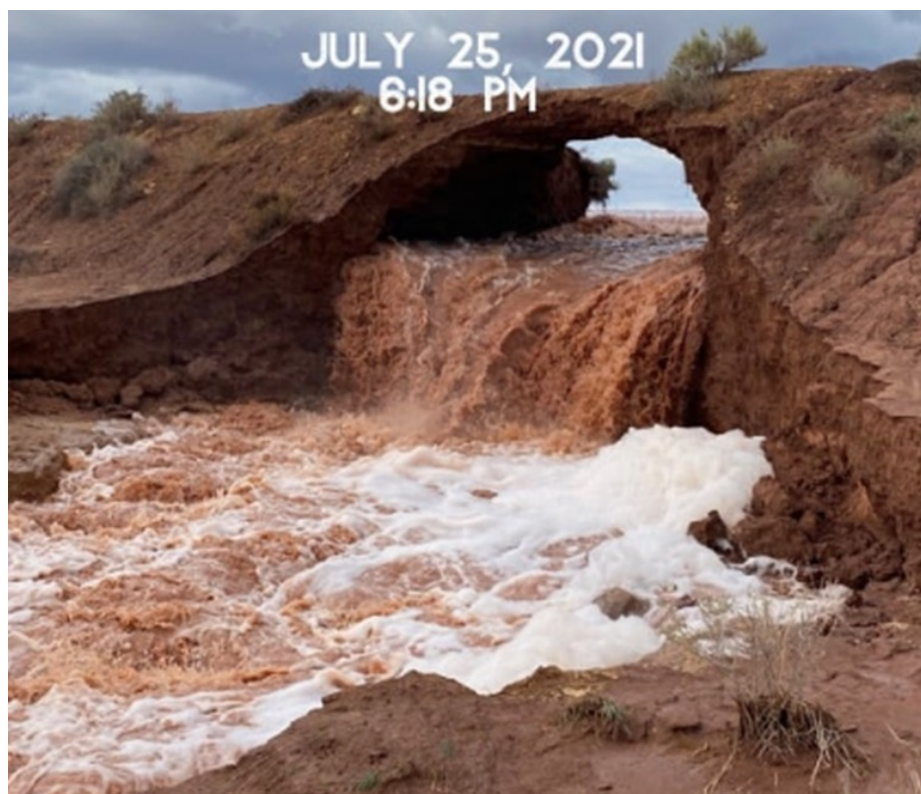
Photo 2: MILLET SWALE DAM FAILURE, JULY 25, 2021
