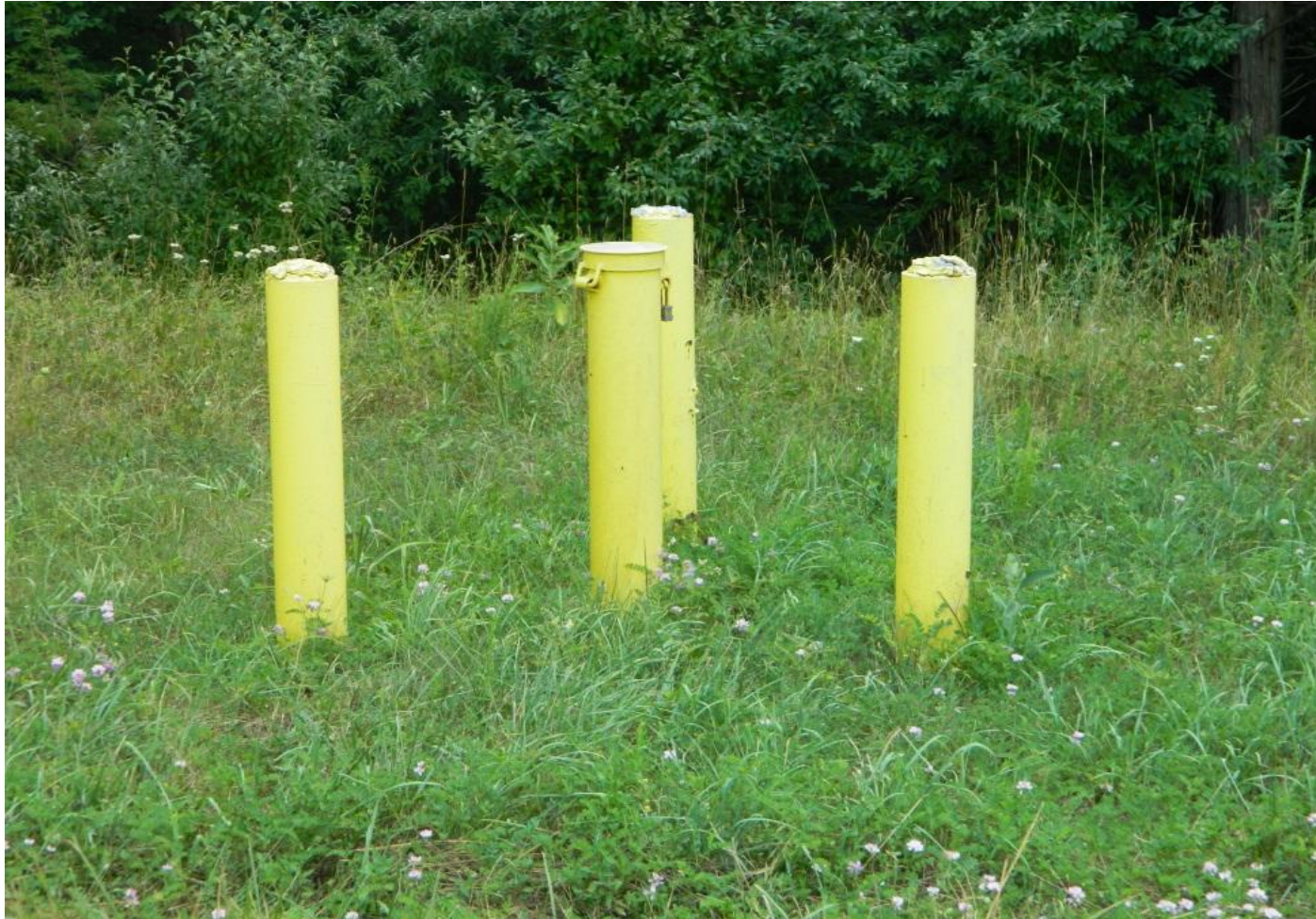
Landfill gas monitoring probe
