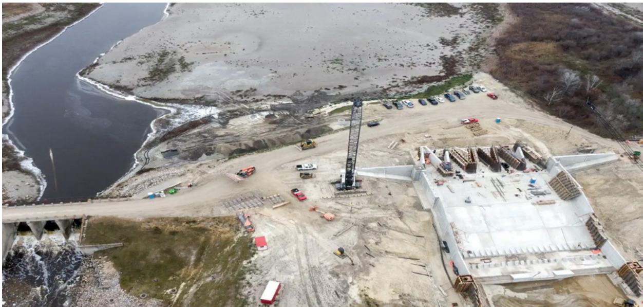
FIGURE 4: AN AERIAL VIEW OF THE LAKE BRONSON DAM REPLACEMENT PROJECT UNDER CONSTRUCTION
