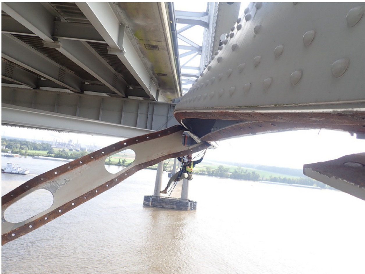
Figure 6: Inspector assessing damage to a truss bottom chord on the Sunshine Bridge over the Mississippi River in Donaldsonville, La., after the impact of an overheight vessel in 2018
