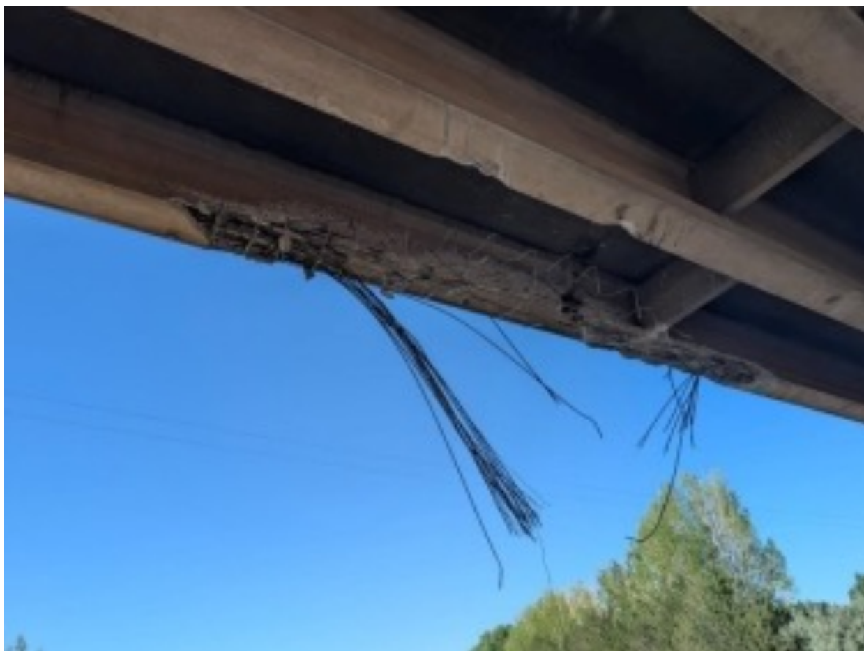
Figure 7. Bridge Strike August 5th, 2025 near Blackfoot, Idaho
