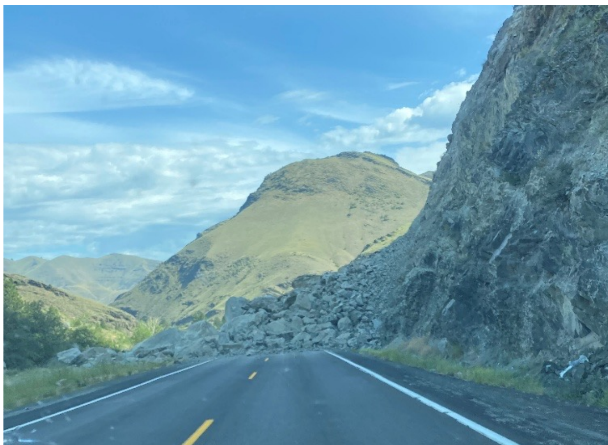
Figure 8. 2020 Rockslide on US 9
