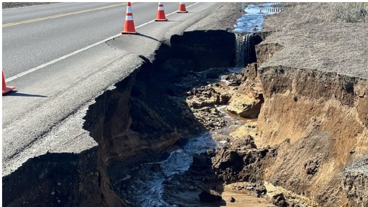
Figure 9. 2023 washout on SH 55
