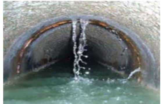
FIGURE 3. Example of Sanitary Sewer Infiltration
