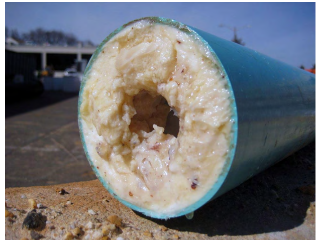
FIGURE 7. FOG buildup in PVC pipe in Huntsville, TX
