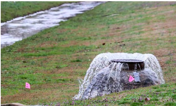
FIGURE 4. Example of Sanitary Sewer Overflow residential or commercial developments.
