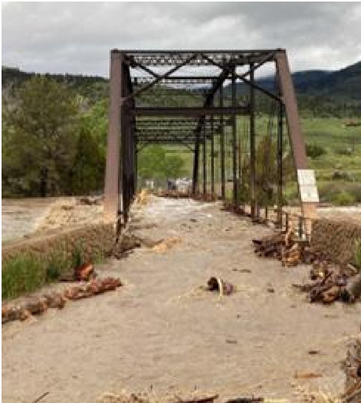
FIGURE 8. 2022 MONTANA FLOOD - CARBELLA BRIDGE OVER YELLOWSTONE RIVER
