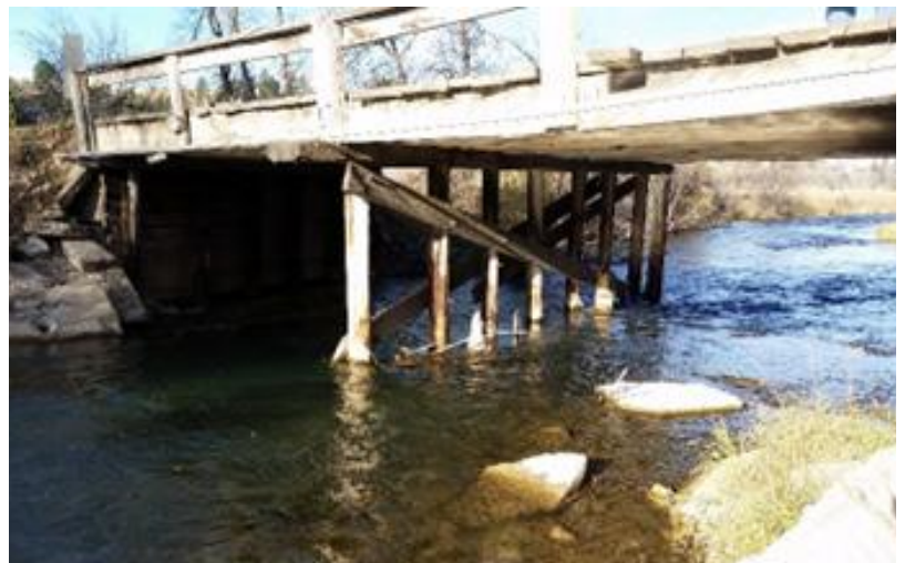
FIGURE 2. TYPICAL TIMBER BRIDGE IN POOR CONDITION
