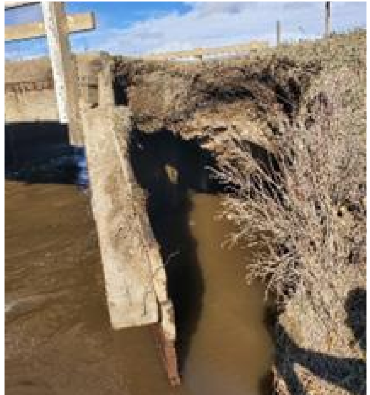
FIGURE 9: FLOOD WATERS ERODE BRIDGE BACKFILL
