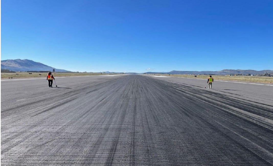
A PAVEMENT CONDITION INDEX (PCI) SURVEY BEING CONDUCTED AT CRATER LAKE-KLAMATH REGIONAL AIRPORT IN KLAMATH FALLS, OR (Photo courtesy of GRI)
