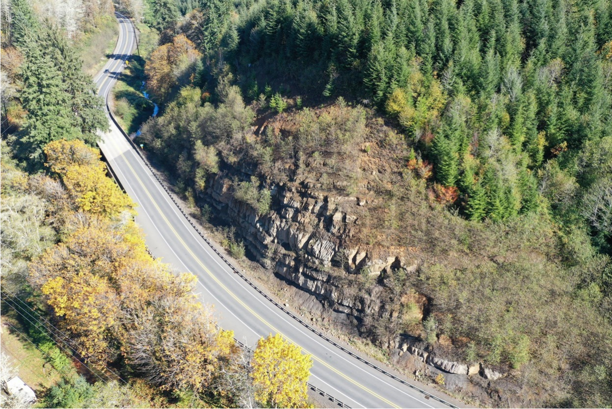
A STABILIZED ROCK SLOPE ALONG U.S. ROUTE 20 NEAR EDDYVILLE, OR (Photo courtesy of Blaine Wruck)
