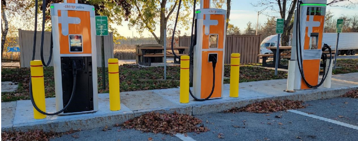
Chargepoint EV chargers at Kennebunk Northbound Service plaza on I-95
