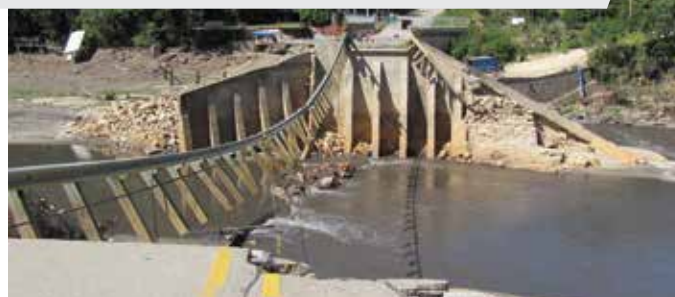
Failed Lake Delhi Dam Embankment in 2010.
