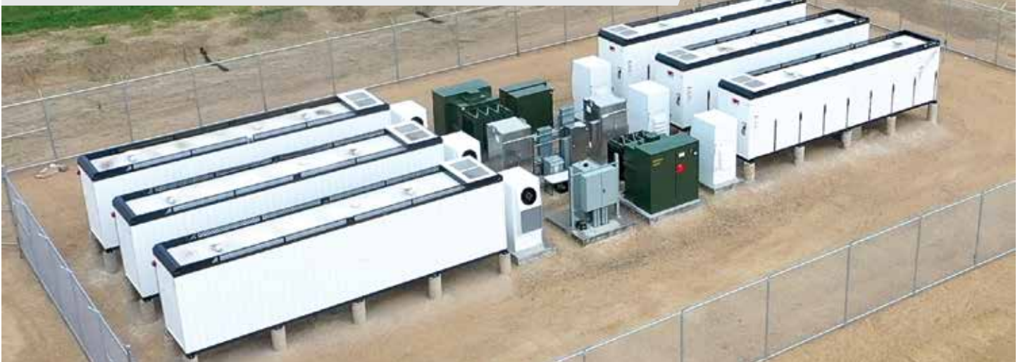
New Cedar Rapids Battery Project Powers Renewable Energy Growth
